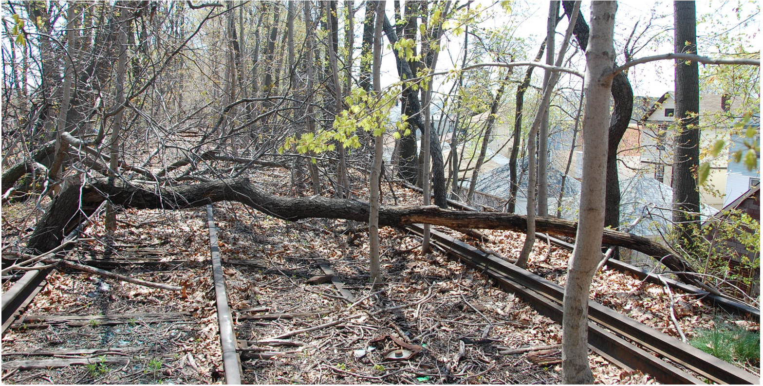
Along the course of the right of way, washouts, crumbling trestles, broken and rusted rails, overgrown vegetation and illegal dumping contribute to the line's dilapidated condition.
